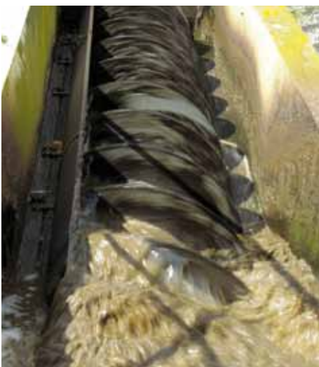
An "Archimedes screw" is used to lift the water into the purifying plant.
