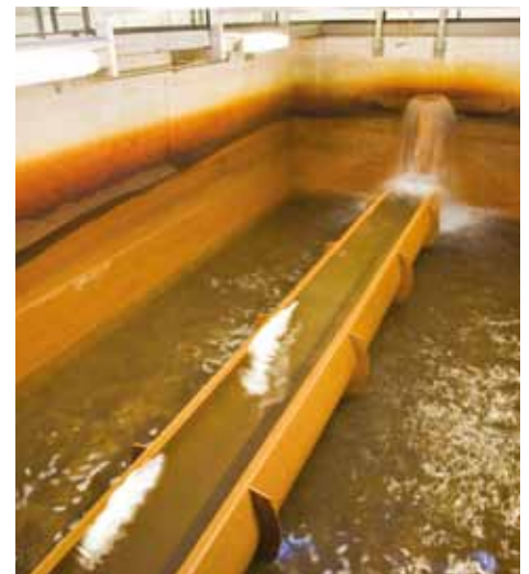
Filtering groundwater. Sand filters trap iron and manganese.
