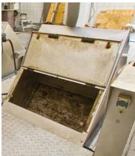
Mechanical purification, where screens trap all bigger items.
